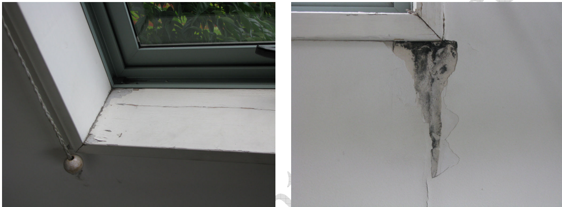
Damage caused by Condensation
